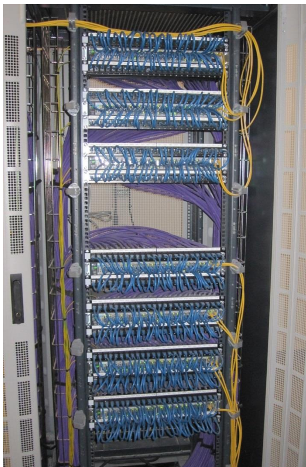
Figure 4. Cabinet layout after patching with 0.25m patch leads, showing groups of two 1U 24-port Cat.6A patch panels, located above and below a 48 port PoE switch. Note gaps left to facilitate maintenance and airflow. Note also the dressing of the infrastructure cables to facilitate the switch installation.
